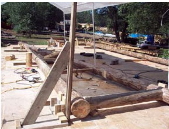
Wooden forms hold the truss at the correct angle while it is constructed
