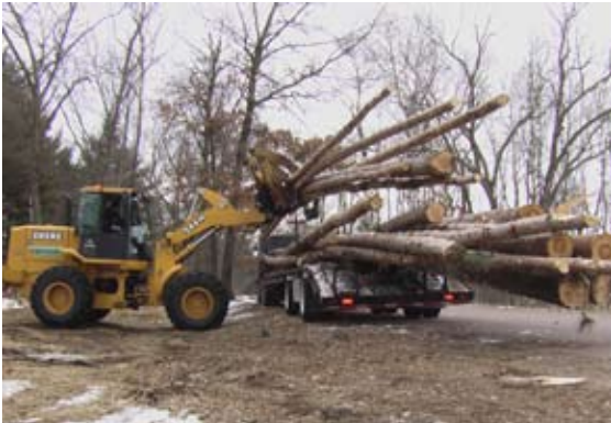
Luther Farms transports the 70-foot logs from the Leopold Shack to the building site
